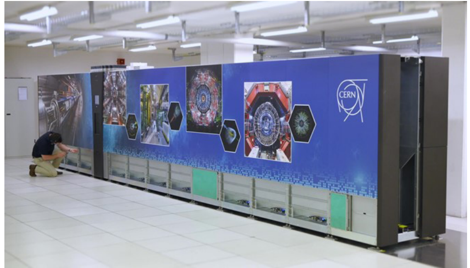
CERN's first Spectra TFinity ExaScale Tape Library was installed in August 2020.
