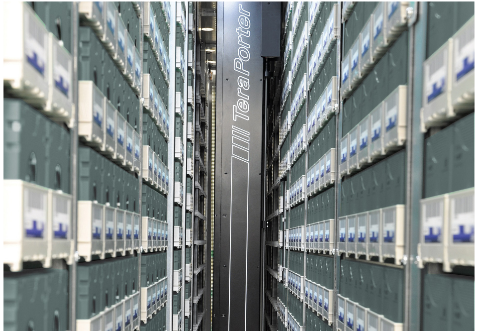
A Spectra TFinity ExaScale Tape Library with LTO-9 media. Instead of individual tape slots, the TFinity tape library has shelves of TeraPack containers that enable higher tape storage density in a smaller footprint.
