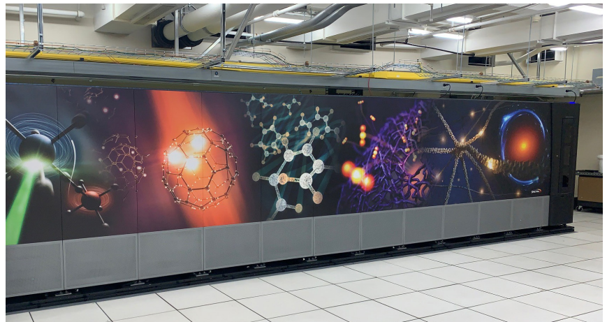
The newly installed 18-frame TFinity ExaScale Tape Library.
